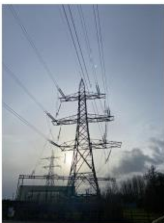
National Grid Sellindge Substation
